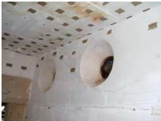
Fig.2b Around Burner
