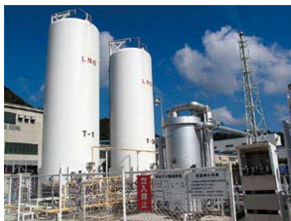
Fig. 2 LNG storage tanks and supply equipment.
