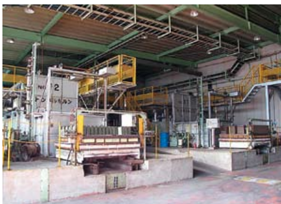
Fig. 1 Inlets of tunnel kilns.
