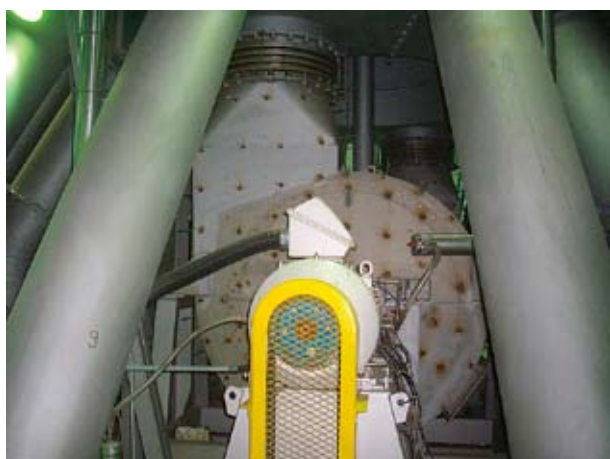
Fig. 8 Hot circulation blower.
