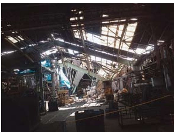
Fig. 2 Plant building seriously damaged by broke down chimney.
