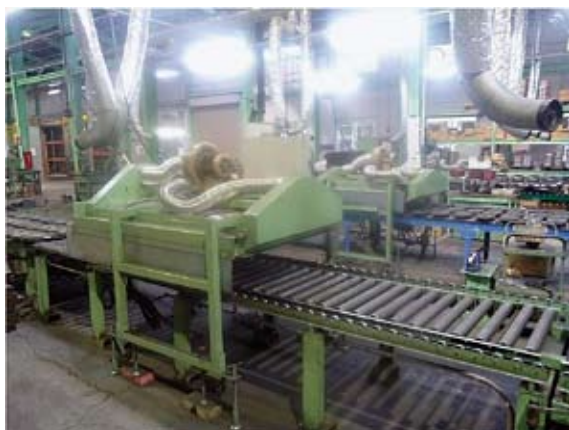
Fig. 4 New quick electric dryer equipped for the SV plate furnishing line.
