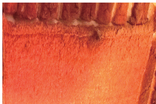
Fig.7 Appearance of coated alumina-fibrous blocks under the dispersal conditions of iron-oxide scale for 8 months in a re-heating furnace.
