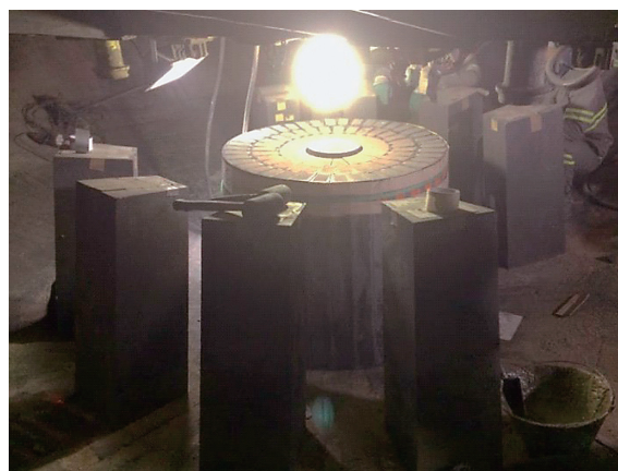
Fig.4 Installation of Mono-block type MHP.
